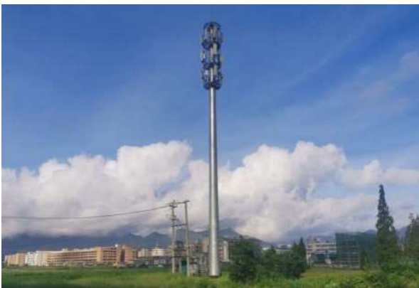
Communication Base Station
