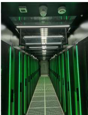
A data center in Shanxi
