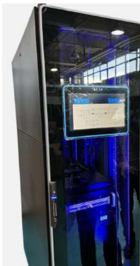
A data center in Hong Kong
