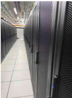
A data center for a communications industry in Taiwan
